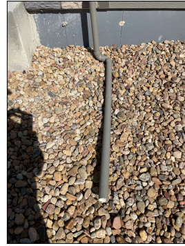
Sump pump discharge line on the south side of the home
