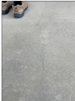
Typical expected cracking noted
