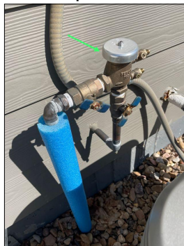
Irrigation back flow device noted as in place and an approved device
