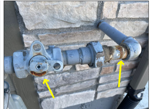
Corrosion / rust on the gas supply lines is a concern
