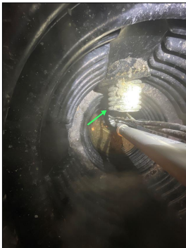
Foundation perimeter drain ports into the sump pump
