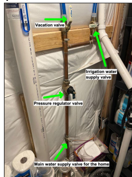
Main water supply entrance to the home is located in the basement storage room
