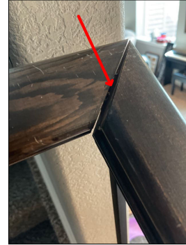
Hand railing joint is separating
