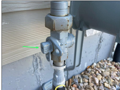
Main gas supply valve for the home
