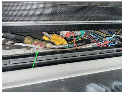
Gas supply valve for the fireplace is located here in the control area, just underneath the firebox
