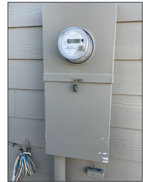
Main panel is located here, on the north exterior wall of the garage
