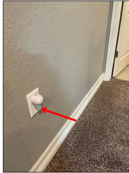
Bottom receptacle has a broken ground plug in it
