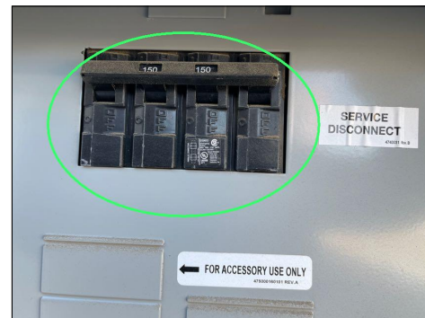
Main electrical service disconnect breaker for the home is located here in the main panel on the north exterior wall of the home
